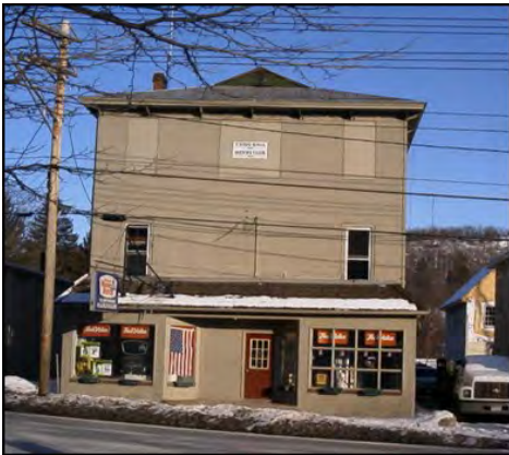
Example of Improper Window Replacement
